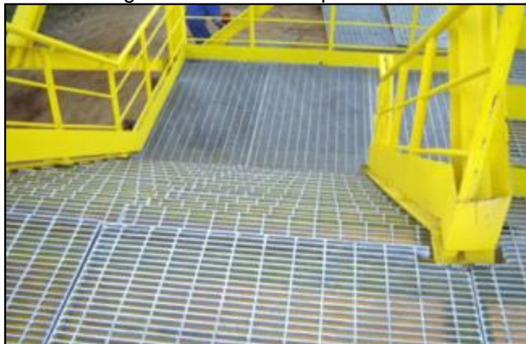
Figura 8 – Grades de piso
